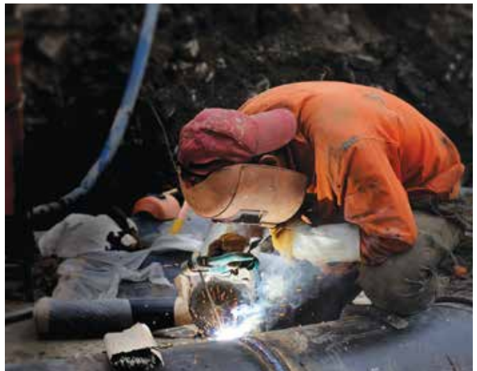
Federal codes regulate the planning, design, operation, maintenance, inspection and testing of pipelines.
